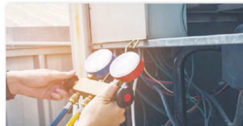
HVRC (REFRIGERATION & AC)
